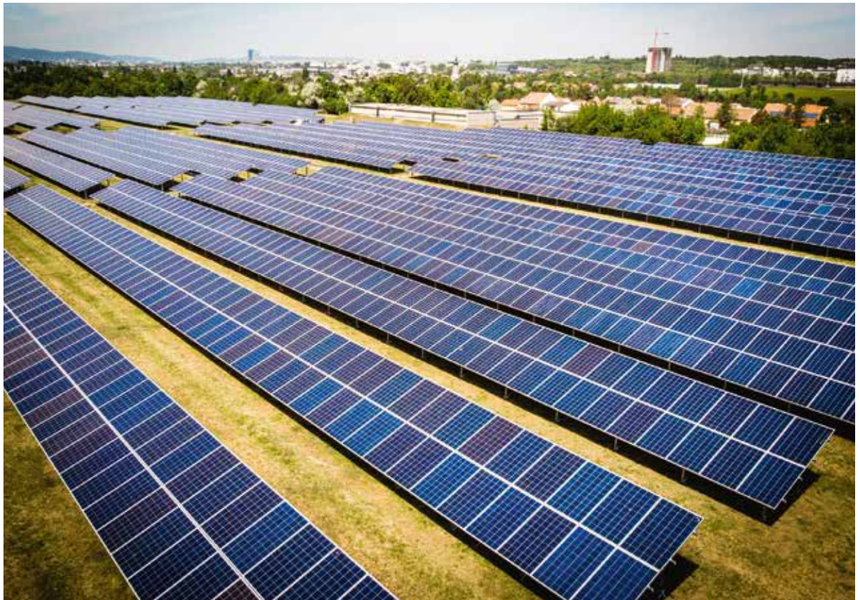
Vienna's largest photovoltaic park in Unterlaa: 6,400 modules covering 28,000 square metres.
