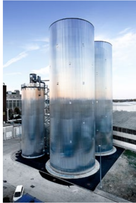
Heating when it is needed: a high-pressure heat storage facility in Vienna's Simmering district.
