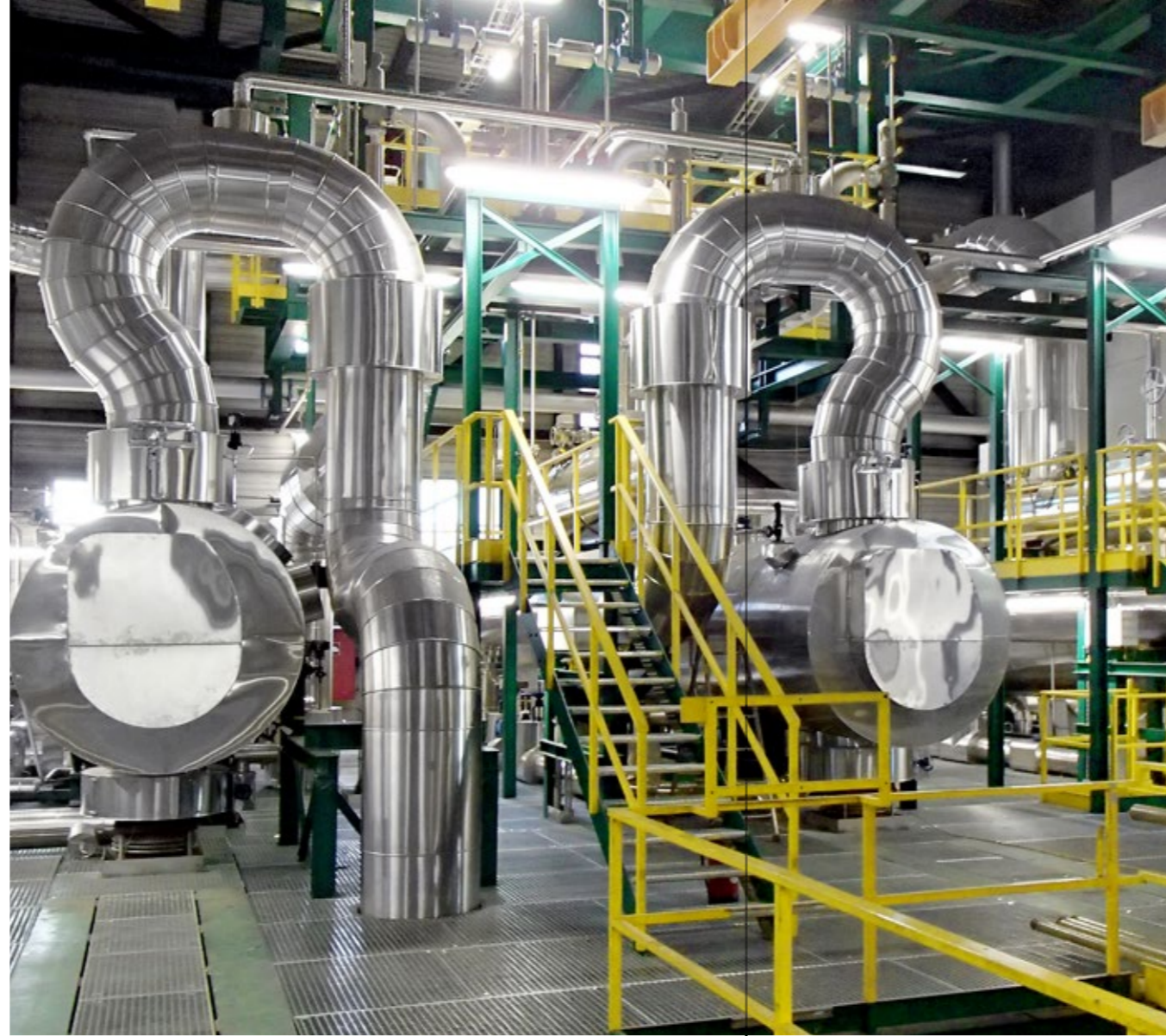
More energy, greater capacity: The Spittelau waste incineration plant was completely renovated at a cost of several hundred million euro.
